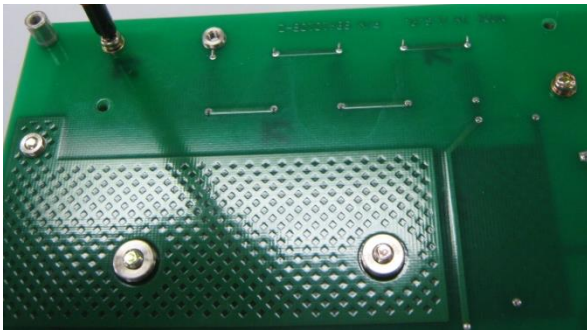
Figure 64 – Removing ozone generator cell assembly
